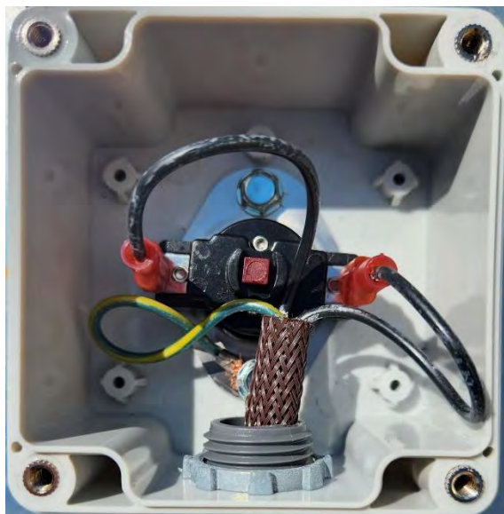
Image 5-16 – Heater housing high-limit switch
