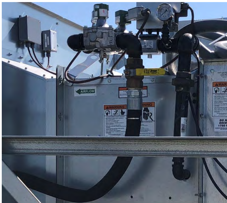
Image 2-8 – Pipe train on NG-fueled heater
