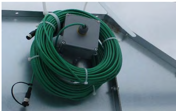
Image 20 – Paddle switch on gravity fill dryer
