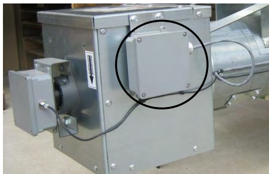
Image 5-3 – Grain discharge chute switch box on auger unload
