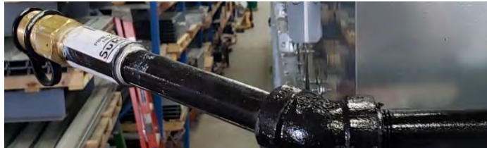
Image 2-11 – End of relief pipe extended past side of dryer
