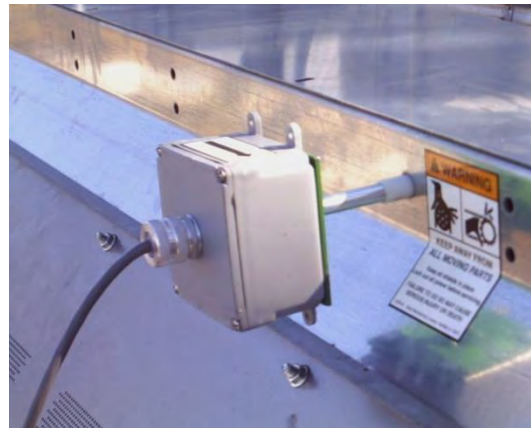
Image 5-6 – Paddle switch T16244 on auger-fill section
