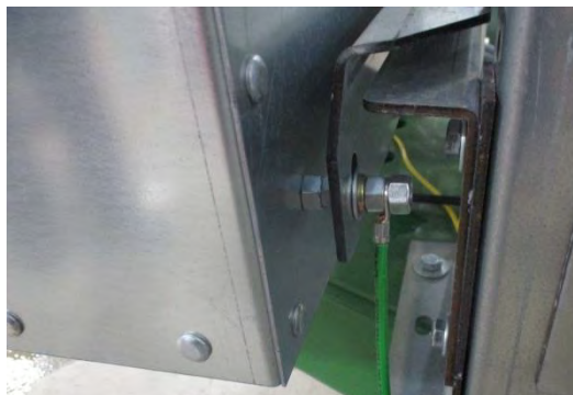
Image 2-21 – Grounding at main power box
