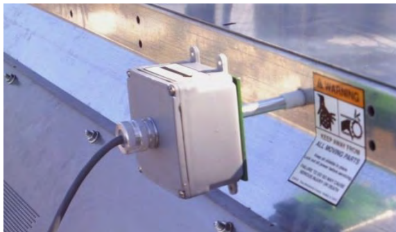
Image 21 – Paddle switch on auger-fill dryer
