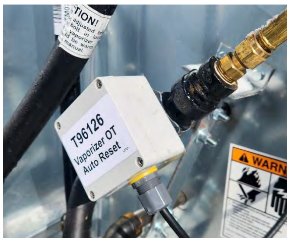
Image 4-13 – Vapor over-temp switch
