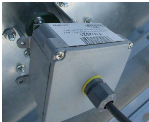
Image 5-5 – Paddle switch T162621 on gravity-fill section
