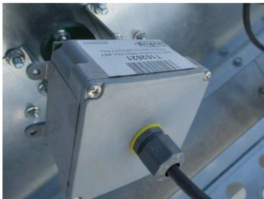
Image 4-31 – Paddle switch T162621 on gravity-fill section
