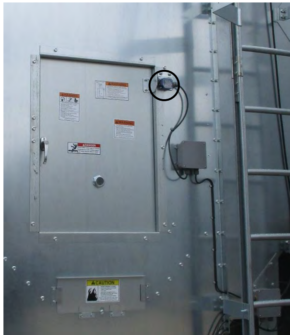
Image 5-13 – Rear door switch & wiring junction box
