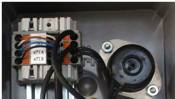
Image 4-23 – Plenum over-temperature switch
