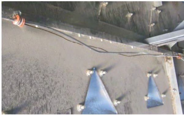
Image 13 – Plenum RTD & over-temp capillary
