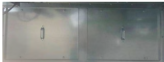
Image 34 – Inlet doors on up-blast fan air intake
