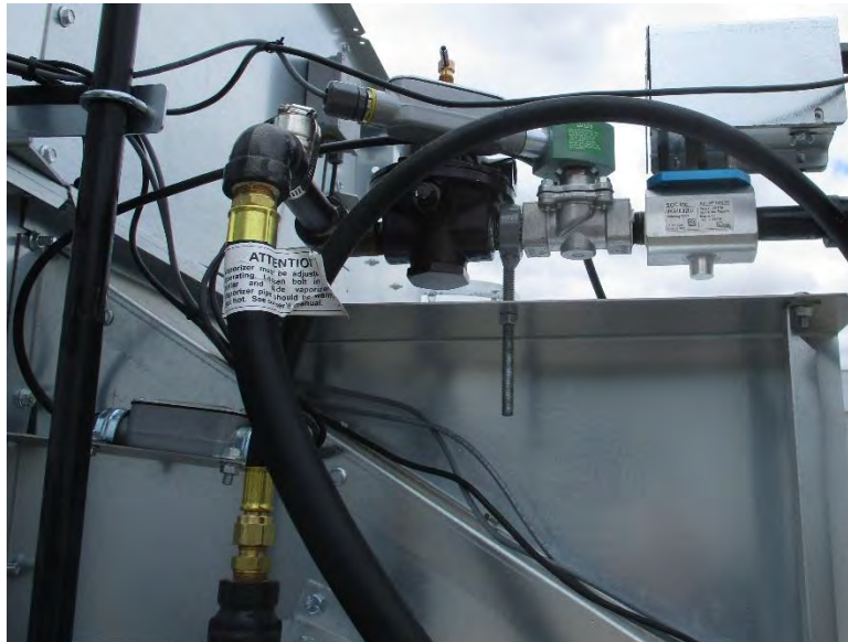
Image 2-7 – Pipe train on LP-fueled heater
