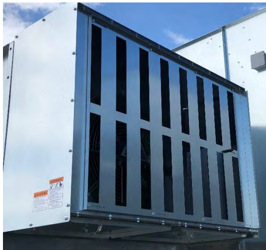
Image 33 – Air inlet louvers
