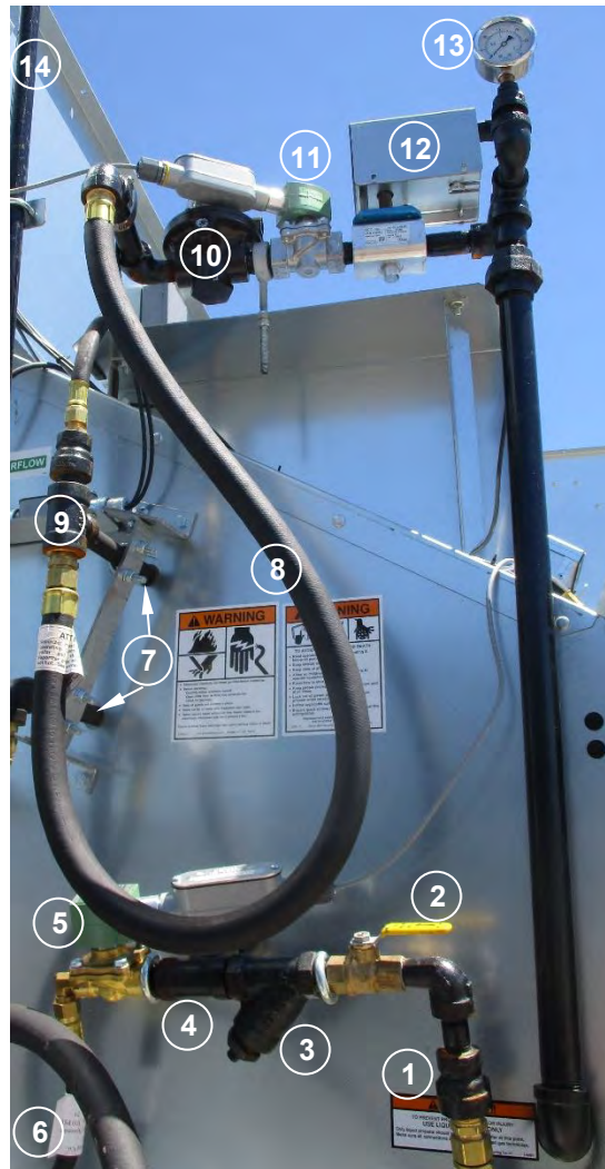
Image 9 – Pipe train components for LP dryer
