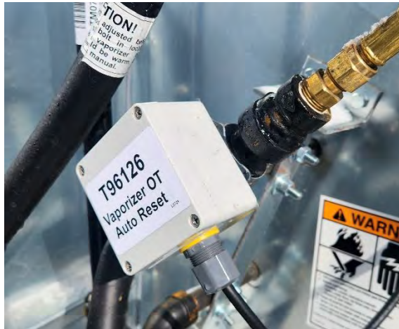
Image 4-13 – Vapor over-temp switch
