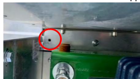
Image 2-17 – Air line entry (circled)
