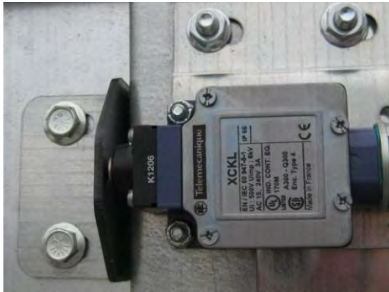
Image 4-12 – Rear door switch
