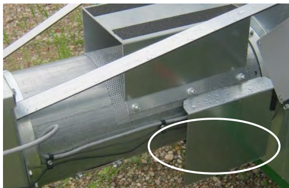
Image 5-23 – Discharge moisture sensor location
