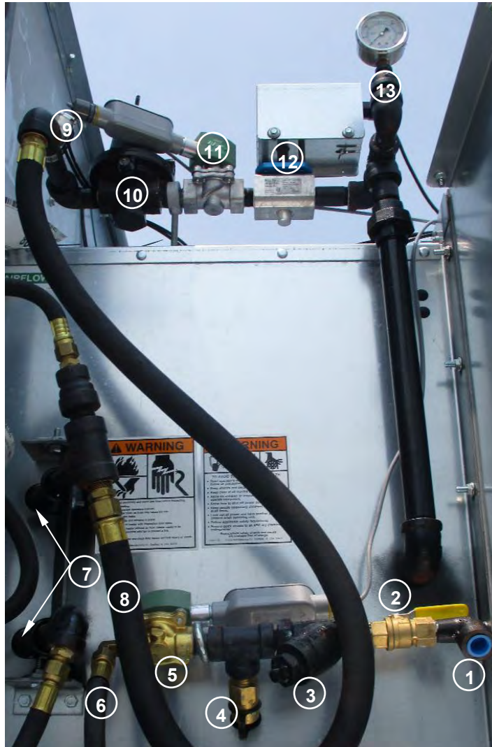
Image 11 – Pipe train components on propane-fueled centrifugal-fan dryer
