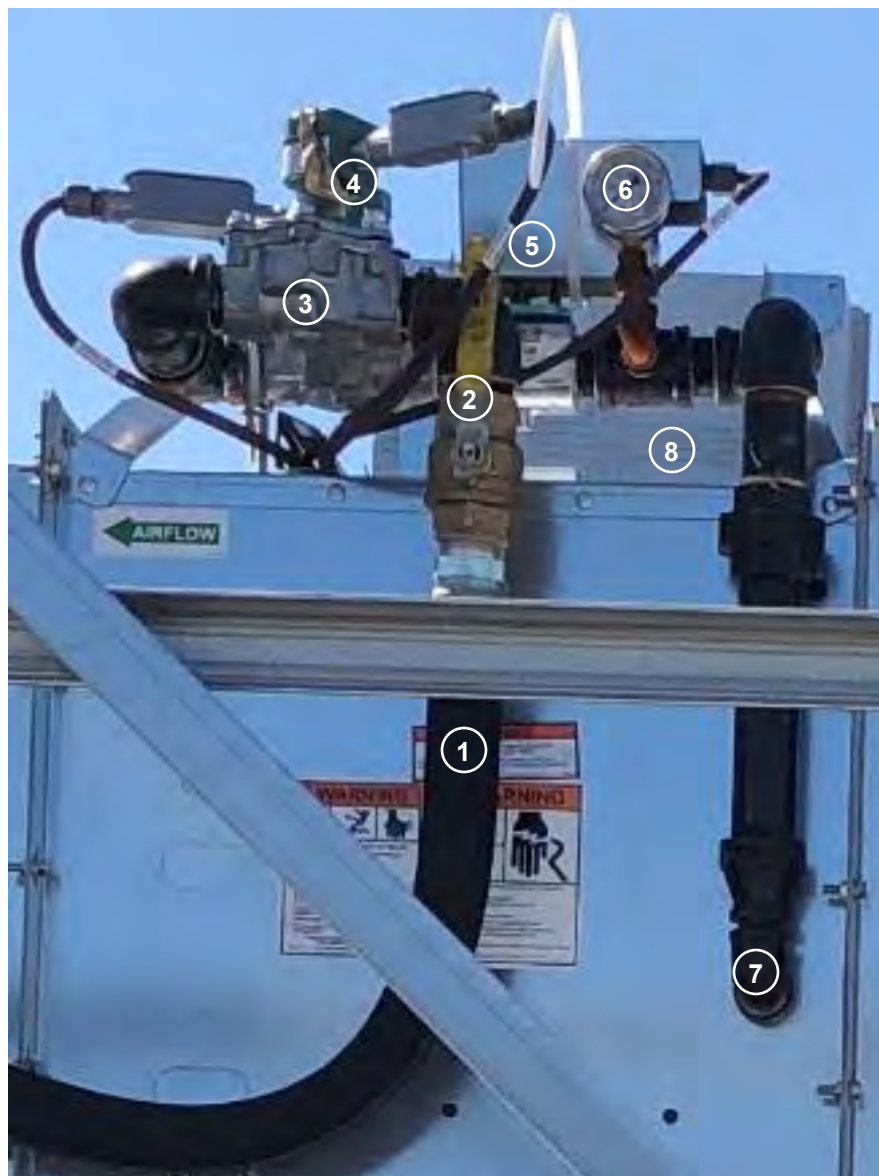
Image 12 – Pipe train components on natural gas-fueled centrifugal-fan dryer
