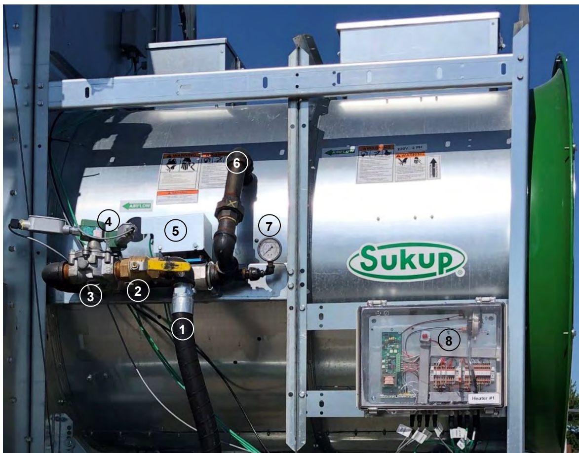
Image 10 – Pipe train components on natural gas-fueled axial-fan dryer
