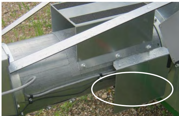
Image 21 – Discharge moisture sensor location
