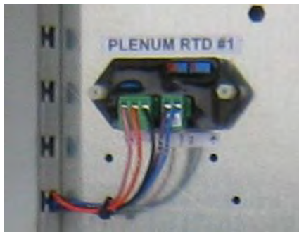
Image 4-16 – Plenum temperature sensor (RTD) transmitter in main power box.
