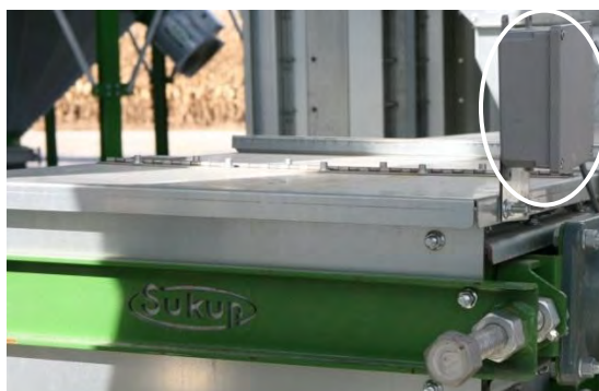
Image 5-3 – Grain discharge chute switch box on drag conveyor unload
