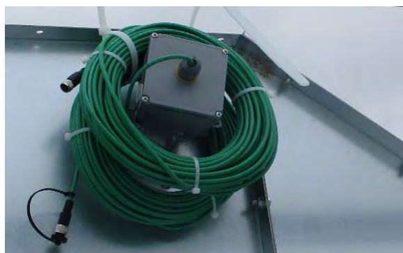
Image 23 – Paddle switch box on gravity fill dryer
