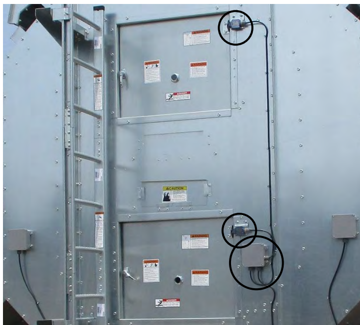
Image 5-11 – Door switches & wiring junction box
