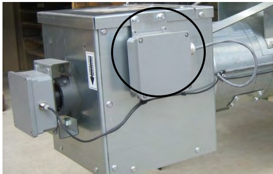
Image 4-5 – Grain discharge chute switch on auger unload system
