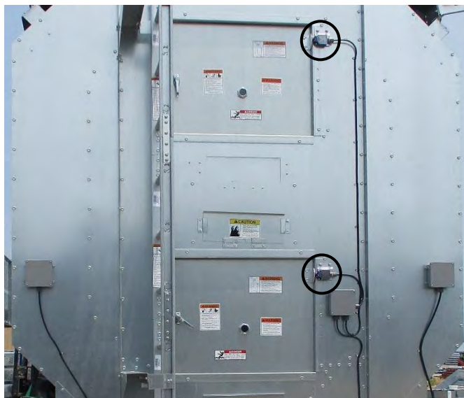
Image 4-35 – Rear access doors & switches
