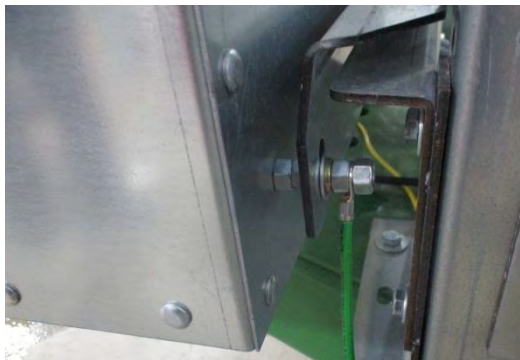
Image 2-4 – Grounding at main power box
