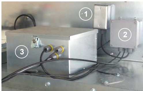
Image 39 – Control boxes above heater housing
