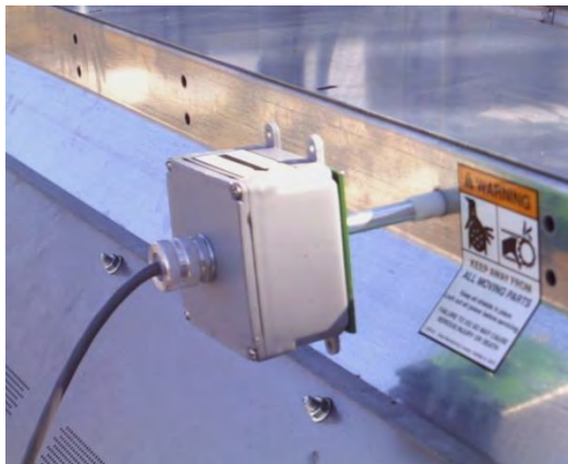
Image 5-5 – Paddle switch T16244 on auger-fill section
