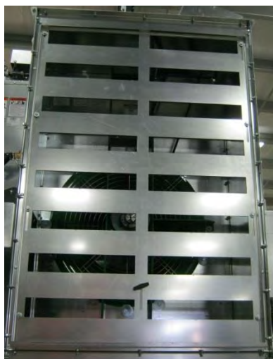
Image 40 – Air inlet louvers
