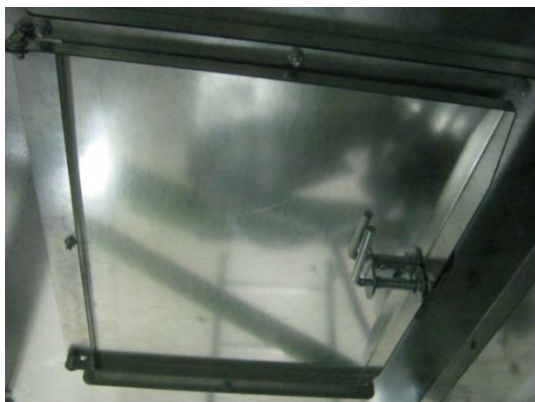
Image 36 – Cleanout door under vacuum-cool duct
