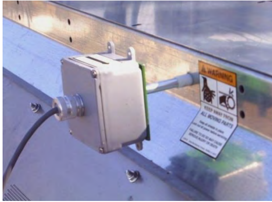
Image 4-28 – Paddle switch box T16244 on auger-load section
