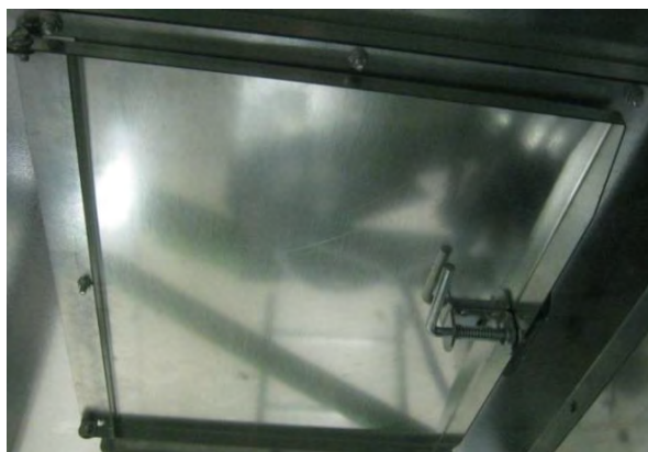
Image 4-46 – Vacuum-cool duct cleanout door (only on centrifugal-fan dryer)
