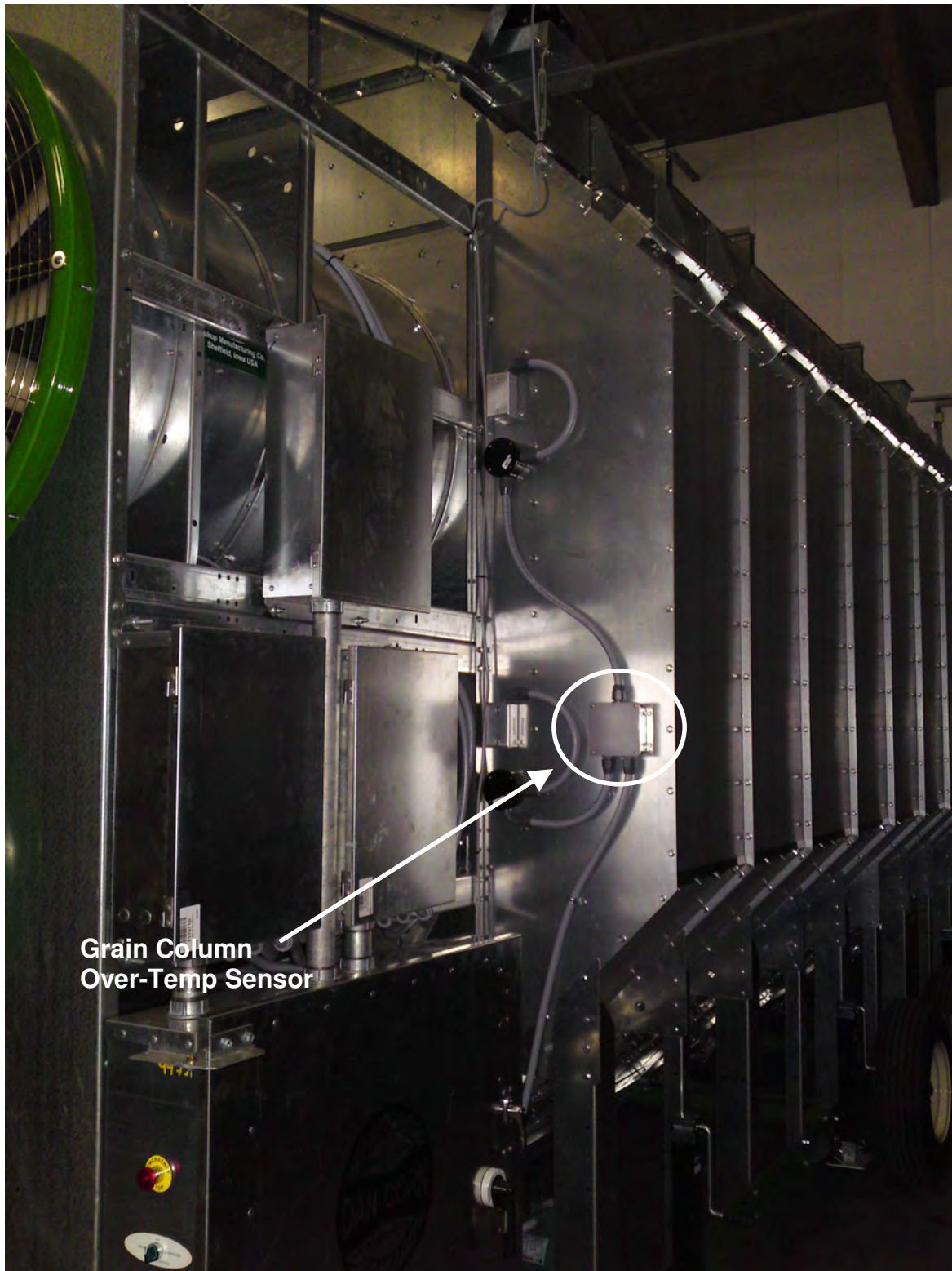
Figure 1.6d: Grain Column Over-Temperature Sensor Installed on Dryer
