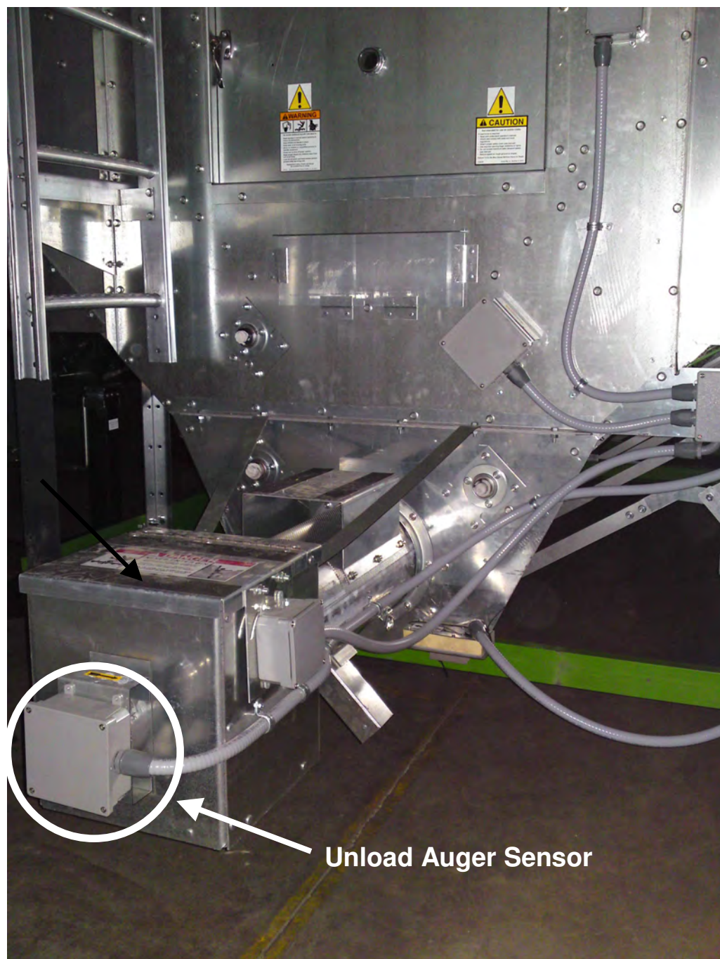
Figure 1.3c: Unload Auger Proximity Sensor Installed on Dryer
