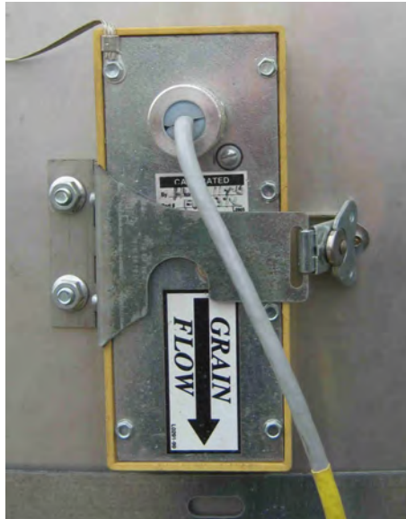
Image 4-9 – Incoming moisture sensor
