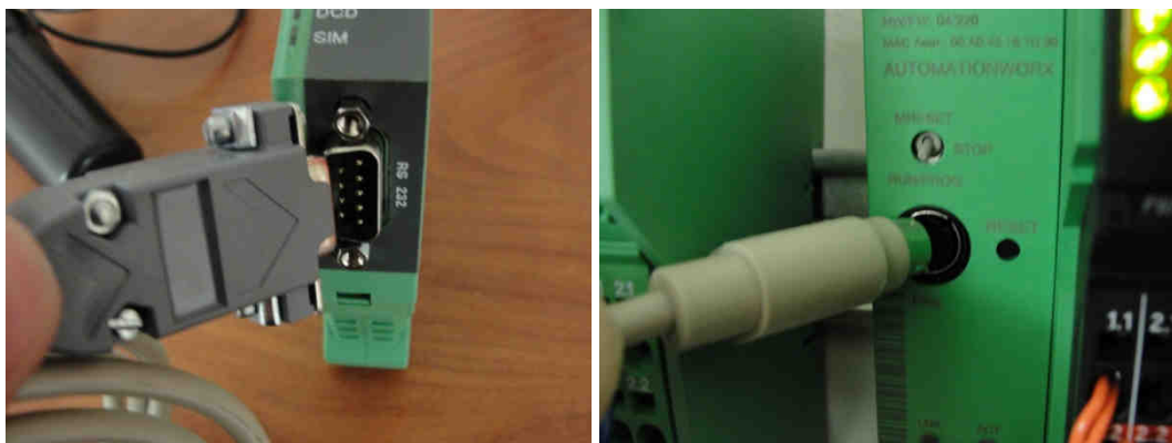
Images 4 and 5 – Connecting modem to PLC
