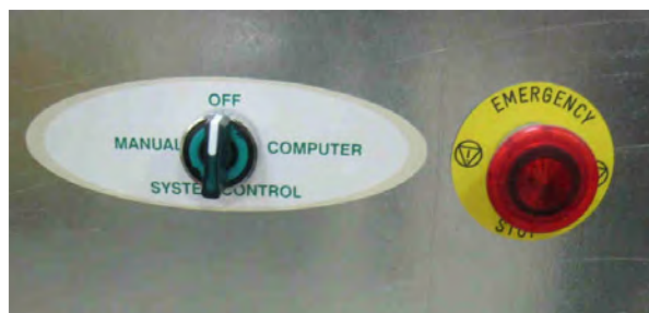
Image 3 – System Control and Emergency Stop switches
