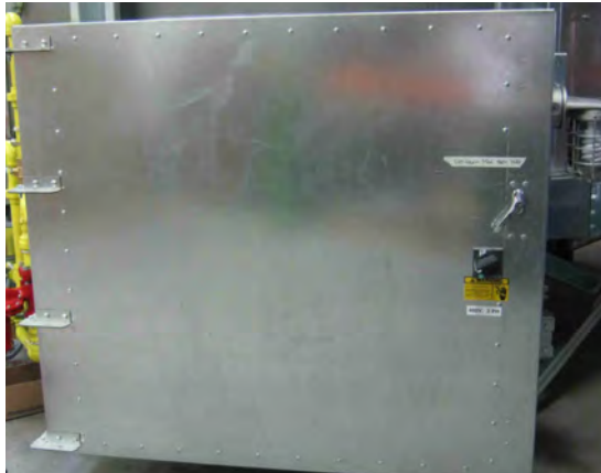
Image 1 – Power distribution box
