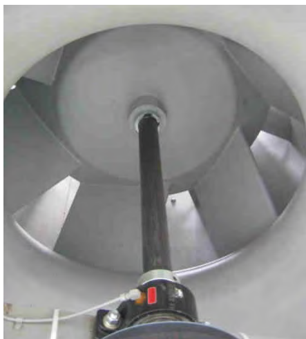
Image 21 – Blower, drive shaft
