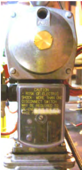
2ND GAS VALVE ACTUATOR WITH REGULATOR
