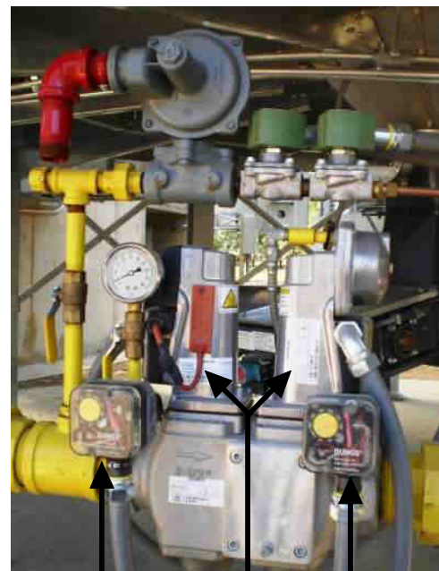
LOW GAS PRESSURE SWITCH MAIN GAS VALVES HIGH GAS PRESSURE SWITCH
