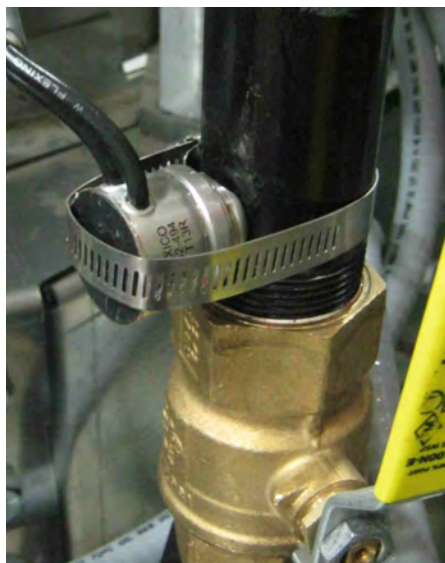
Image 4-4 – Vapor over-temp switch
