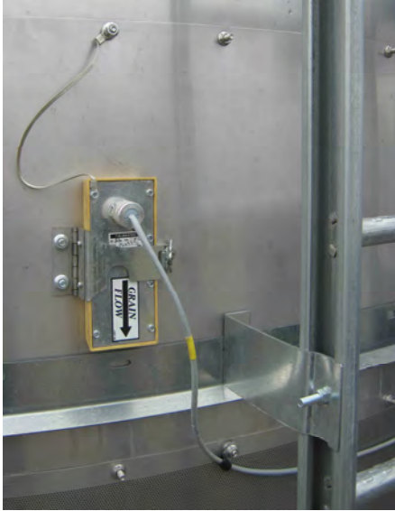
Image 26 – Incoming moisture sensor
