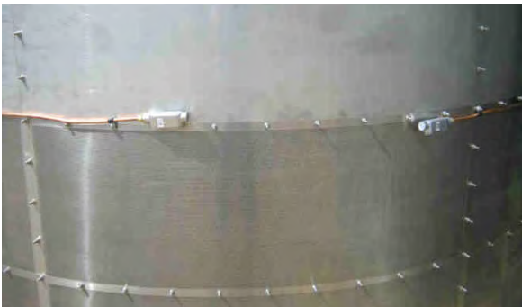
Image 27 – Outside over temperature sensor
