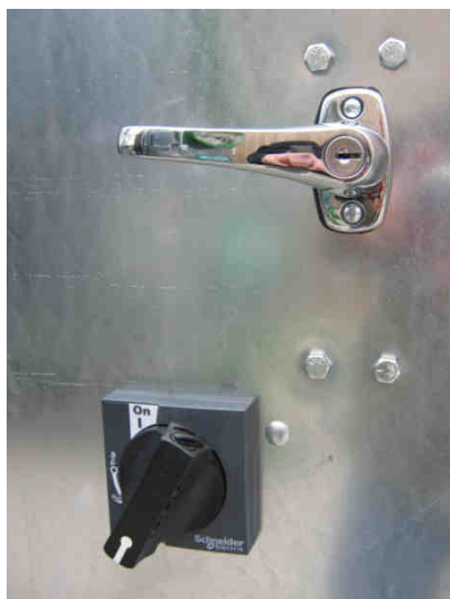
Image 9 – Latch and Main Disconnect switch in “Off” position
