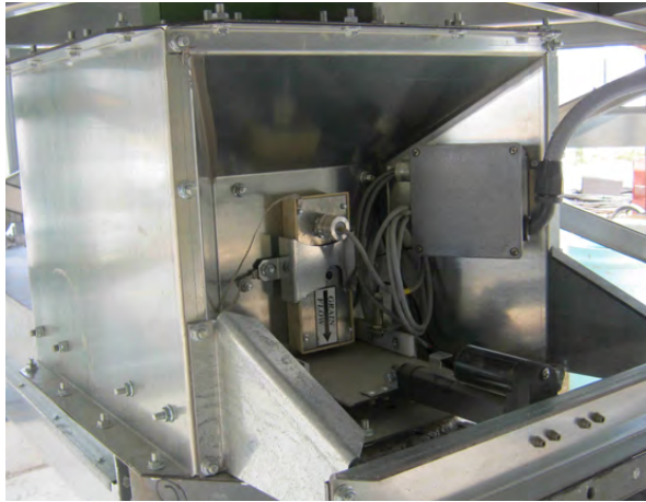
Image 29 – Static moisture sensor
