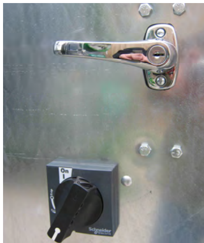
Image 2 – Door latch and Main Disconnect switch
