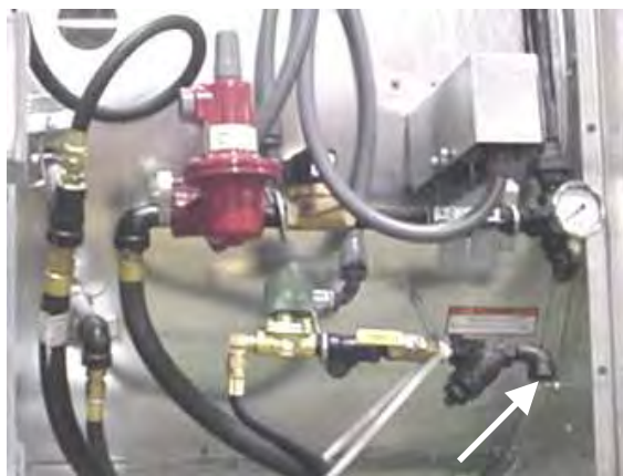
Connection to liquid manifold on Dryer
