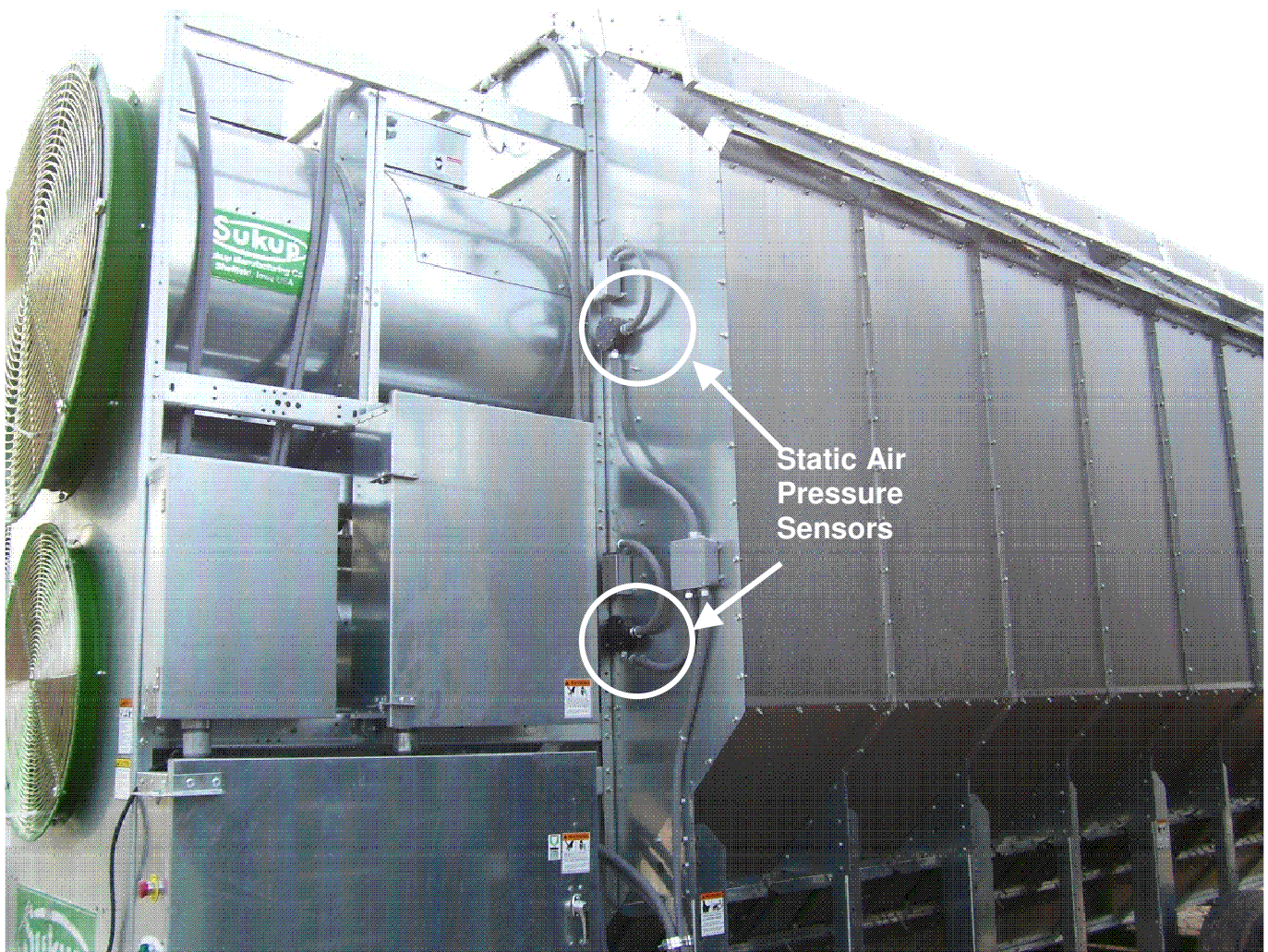
Figure 1.9d: Static Air Pressure Sensors Installed on Dryer
