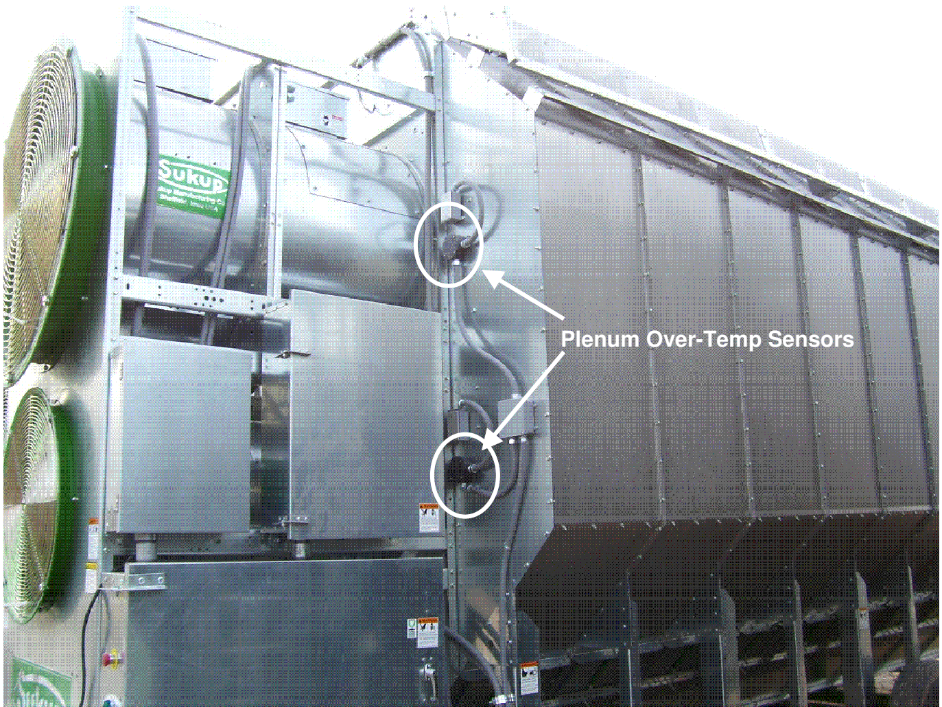
Figure 1.10c: Plenum Over-Temperature Sensors Installed on Dryer
