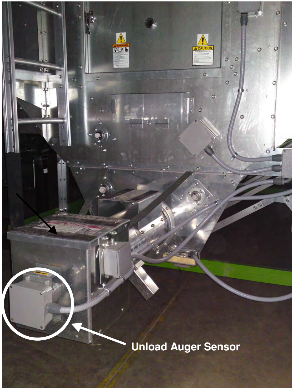
Figure 1.3c: Unload Auger Proximity Sensor Installed on Dryer
