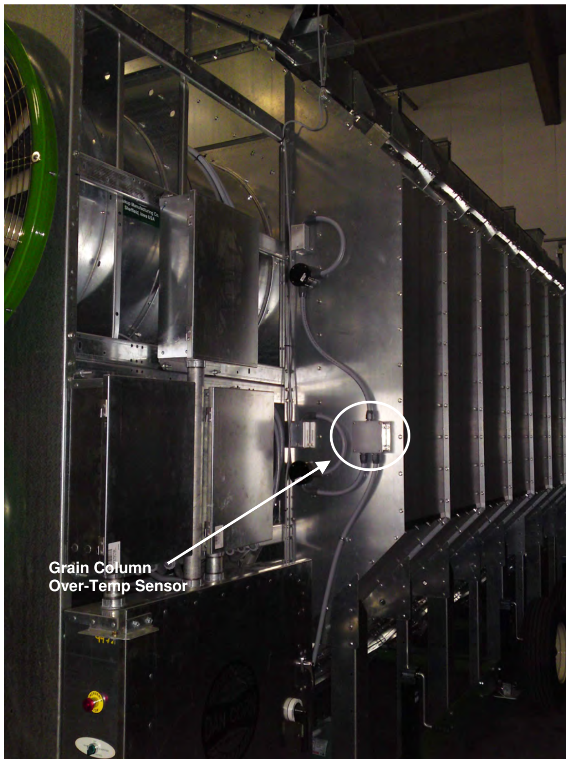
Figure 1.6d: Grain Column Over-Temperature Sensor Installed on Dryer
