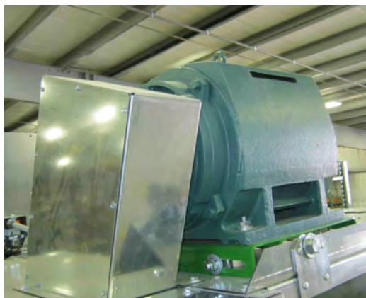
Image 39 – Fan motor and drive shield
