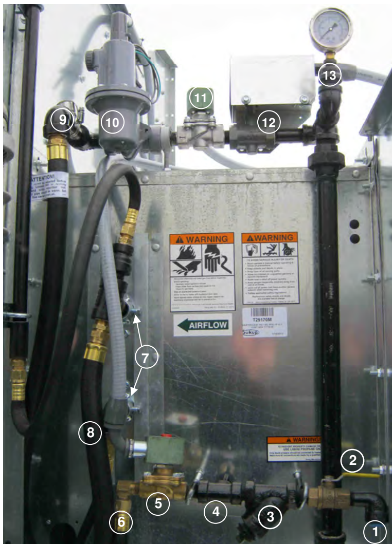
Image 7 – Pipe train components
