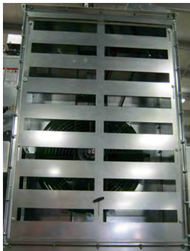
Image 38 – Air inlet louvers
