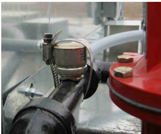
Image 5-9 – Vapor over-temp switch on dryer
