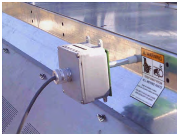
Image 5-5 – Paddle switch box on dryer
