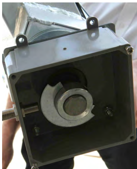
Image 16 – Unload proximity switch mounted on jump auger
