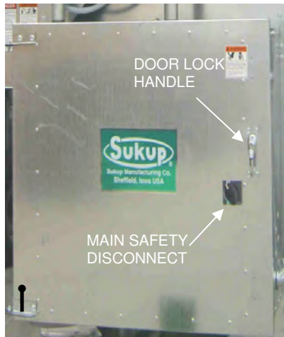
Image 1 – Power distribution box
