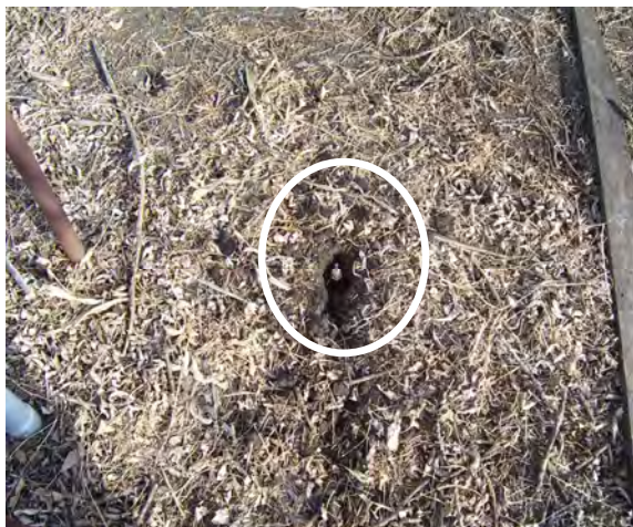
Image 2-5 – Ground rod, buried
