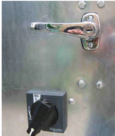
Image 2 – Main safety disconnect
