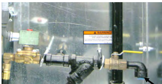
Image 2-1 - LP-fueled centrifugal dryer
