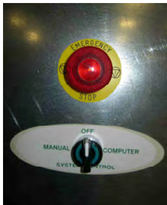
Image 23 – Emergency stop button and system control switch
