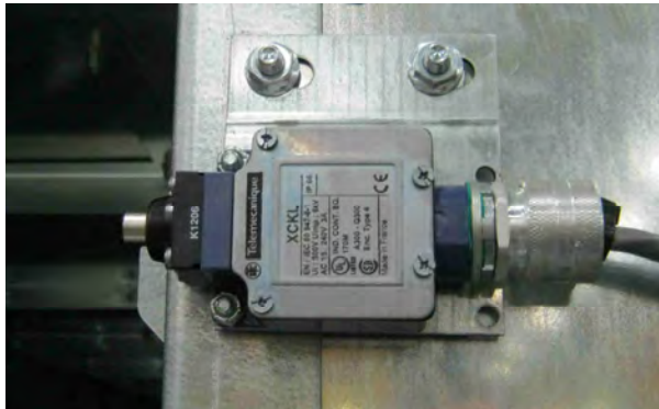
Image 14 – Rear door switch
