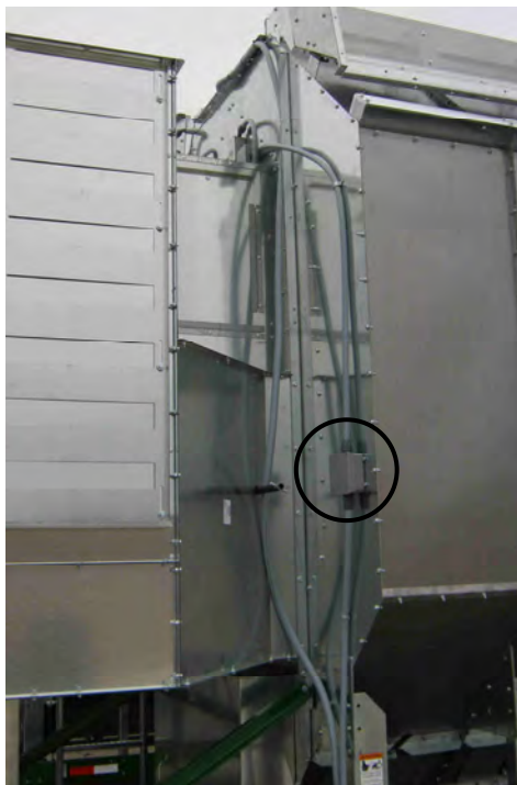
Image 5-13 – Grain column over-temp switch
