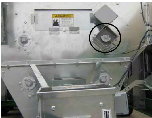
Image 5-16 – Metering roll proximity switch
