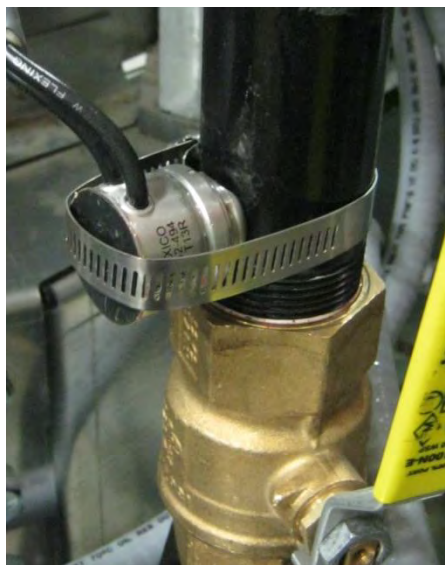
Image 4-4 – Vapor over-temp switch
