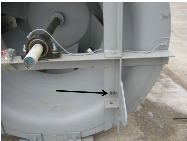
Image 3-6 – Grease zerks for blower shaft bearings
