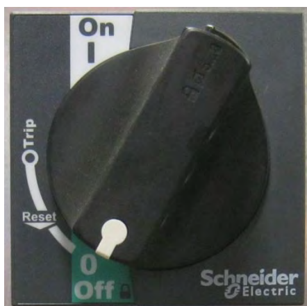
Image 2 – Main Disconnect switch
