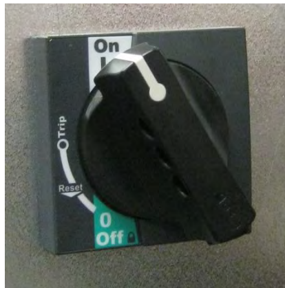
Image 2-2 – Main Disconnect switch
