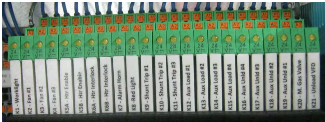
K relays energized by 24VDC from PLC
