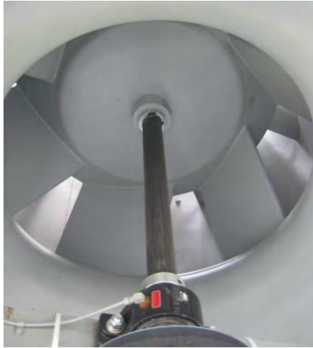
Image 15 – Blower, drive shaft
