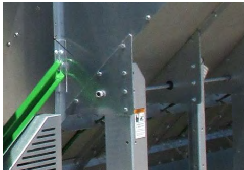
Image 2-15 – Discharge moisture sensor conduit at front of dryer
