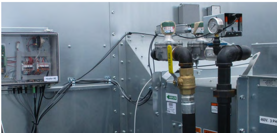
Image 2-8 – Pipe train on NG-fueled heater
