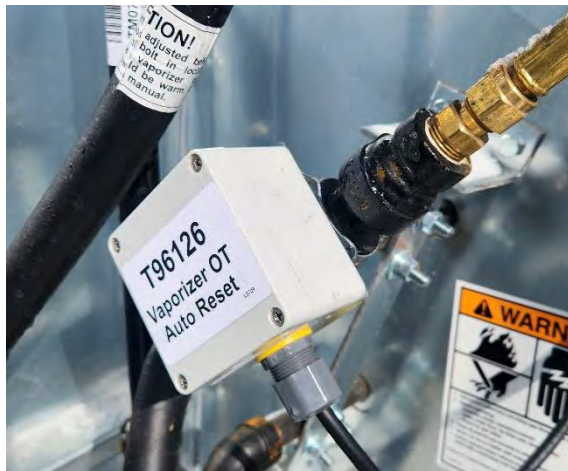
Image 4-13 – Vapor over-temp switch
