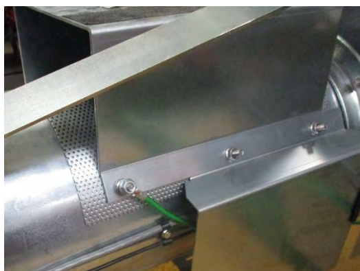
Image 2-23 – Grounding at discharge tube
