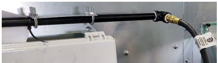
Image 2-12 – Relief pipe attached above heater box
