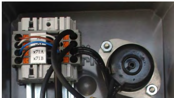
Image 4-24 – Plenum over-temperature switch
