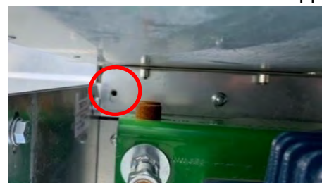
Image 2-18 – Air line entry (circled)
