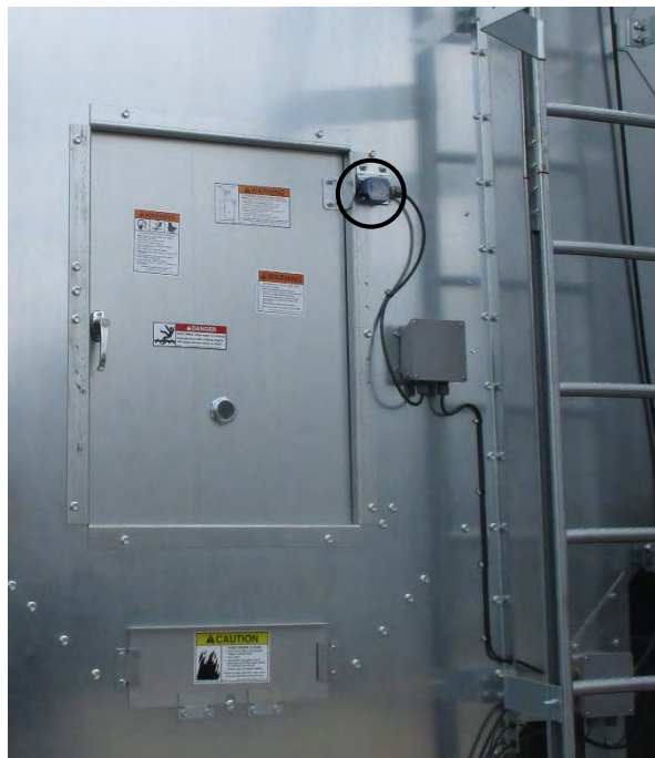
Image 5-13 – Rear door switch
