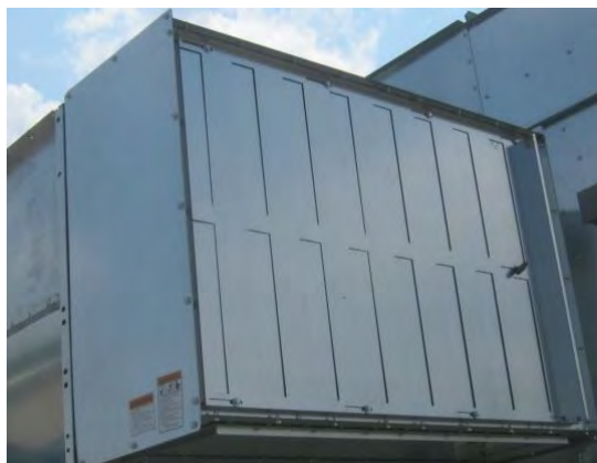
Image 33 – Air inlet louvers
