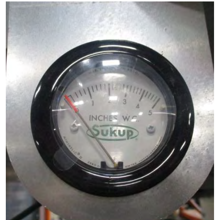
Image 3-3 – Vacuum pressure gauge
