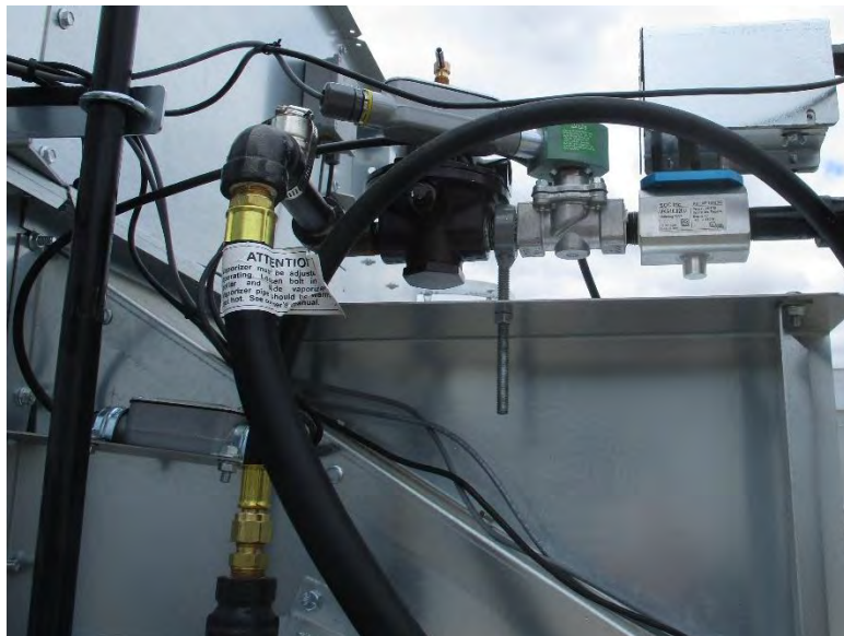
Image 2-7 – Pipe train on LP-fueled heater
