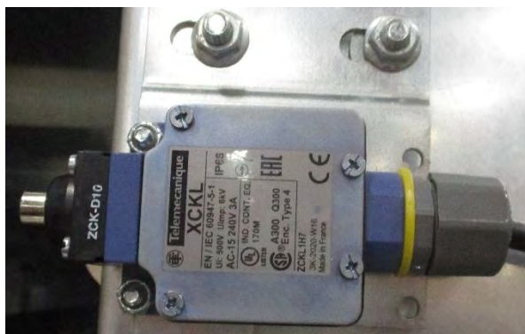
Image 15 – Rear door switch
