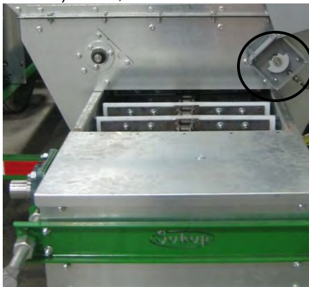
Image 5-18 – Meter roll proximity switch on dryer with conveyor unload
