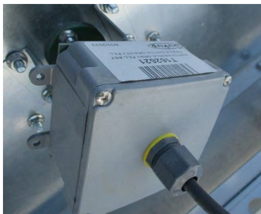
Image 5-5 – Paddle switch T162621 on gravity-fill section
