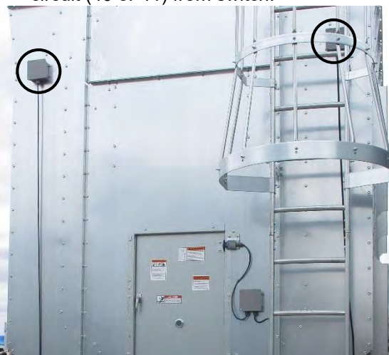
Image 5-15 – Grain column over-temp switches
