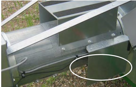
Image 4-2 – Discharge moisture sensor location on auger-unload dryer
