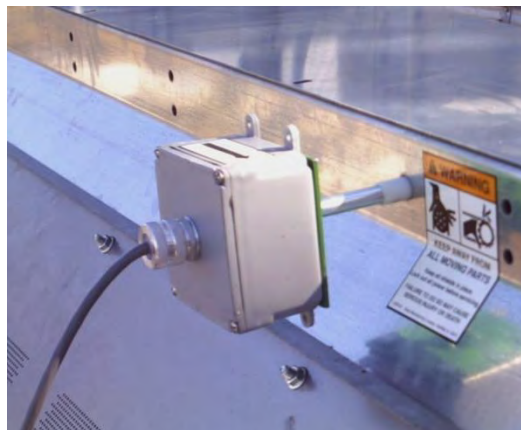
Image 5-6 – Paddle switch T16244 on auger-fill section
