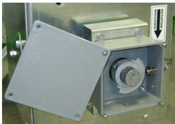
Image 17 – Unload auger proximity switch
