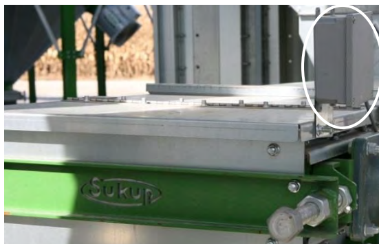
Image 5-2 – Grain discharge chute switch on drag conveyor unload
