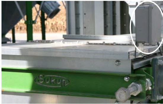
Image 4-29 – Grain discharge chute switch on drag conveyor unload system
