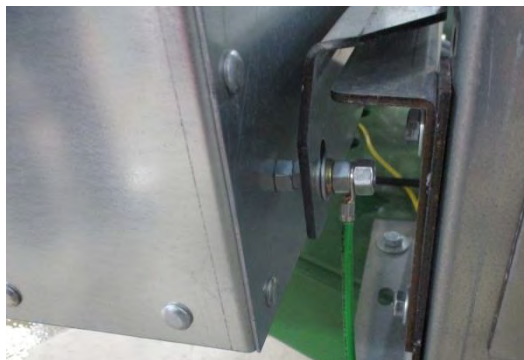
Image 2-22 – Grounding at main power box
