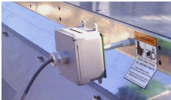
Image 21 – Paddle switch on auger-fill dryer
