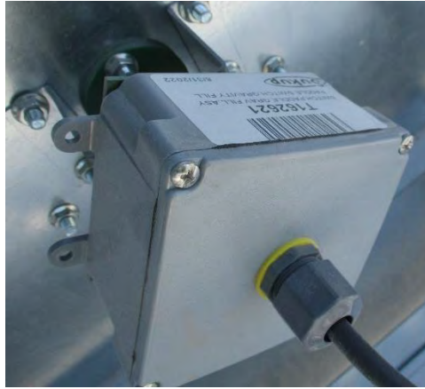
Image 4-8 – Paddle switch T162621 on gravity-fill section
