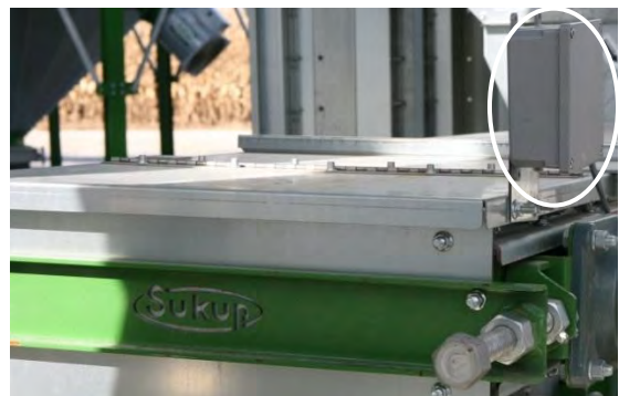
Image 5-3 – Grain discharge chute switch on drag conveyor unload
