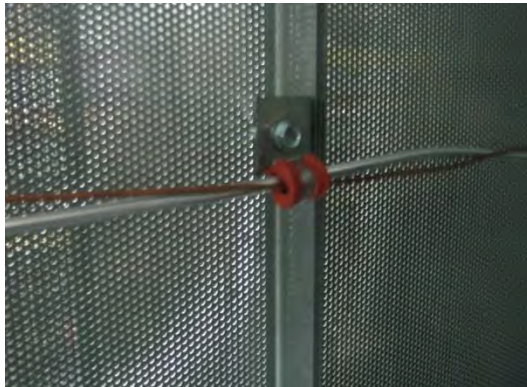
Image 15 – Plenum RTD (silver) and over-temp capillary (copper)
