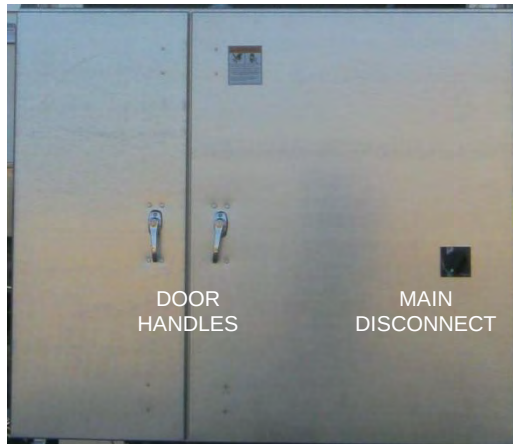
Image 1 – Power distribution box
