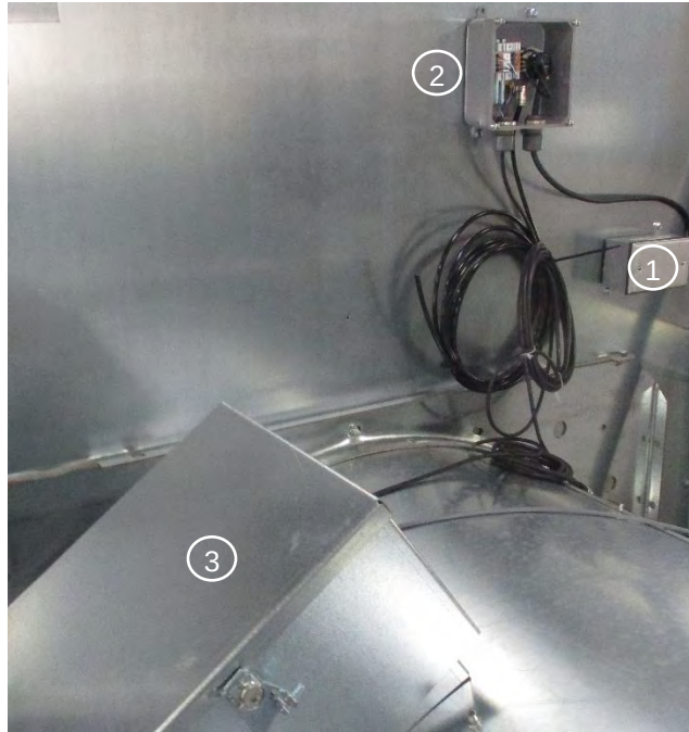
Image 5-19 – Locations on axial dryer of plenum temp sensor RTD, air switch hose, plenum over-temp switch & heater housing high-limit switch
