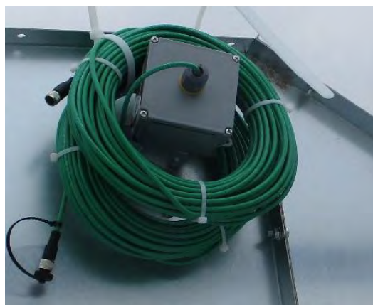
Image 5-6 – Paddle switch on gravity-fill section
