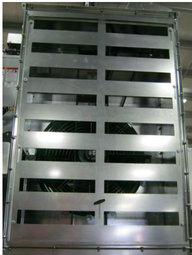
Image 40 – Air inlet louvers
