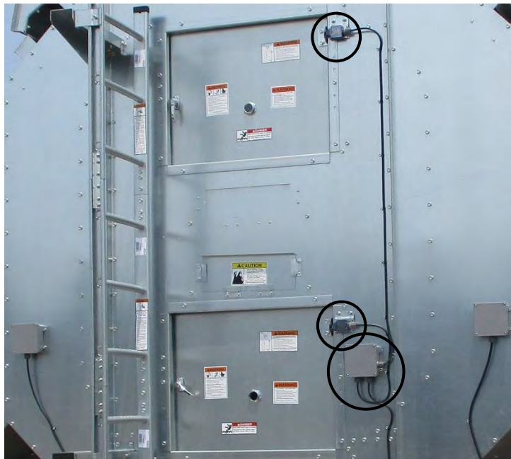
Image 5-11 – Door switches & wiring junction box
