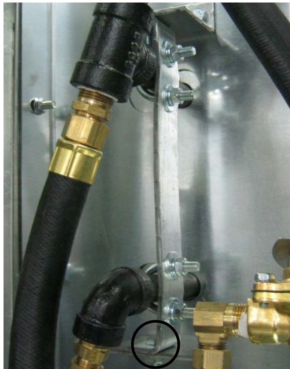
Image 3-2 – Vaporizer bkt. on centrifugal-fan dryer
