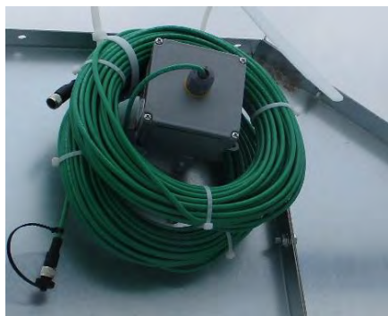
Image 4-9 – Paddle switch T162621 on gravity-fill section
