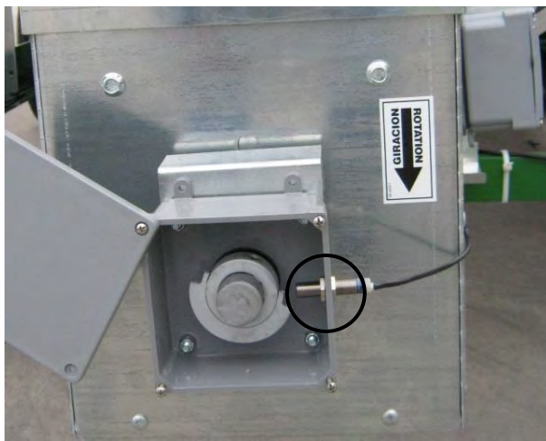
Image 4-10 – Unload auger proximity switch
