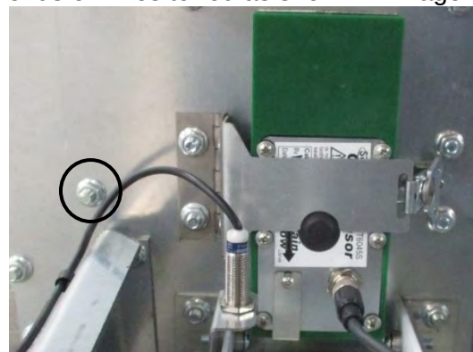
Image 2-6 – Grounding at sample box
