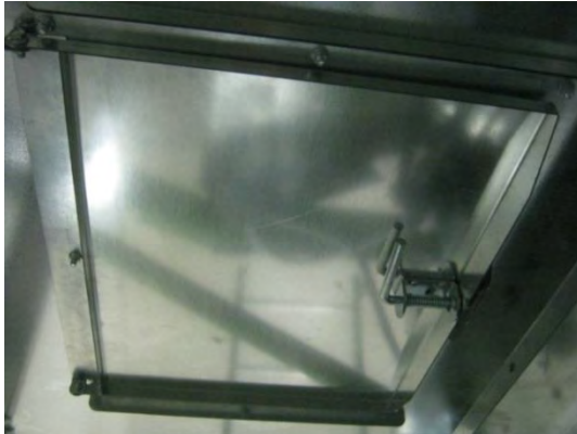
Image 36 – Cleanout door under vacuum-cool duct
