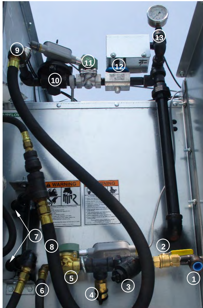
Image 10 – Pipe train components on centrifugal-fan dryer
