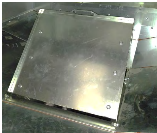
Image 38 – Plenum divider door by burner
