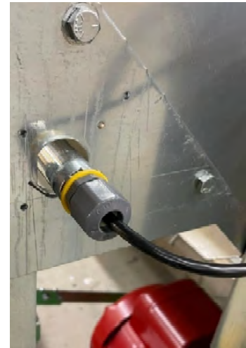
Image 10 - Cable (at front of dryer) from right rear junction box
