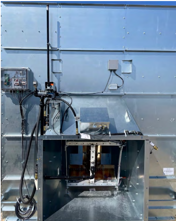
Image 7 - Upper heat section of mixed-flow dryer
