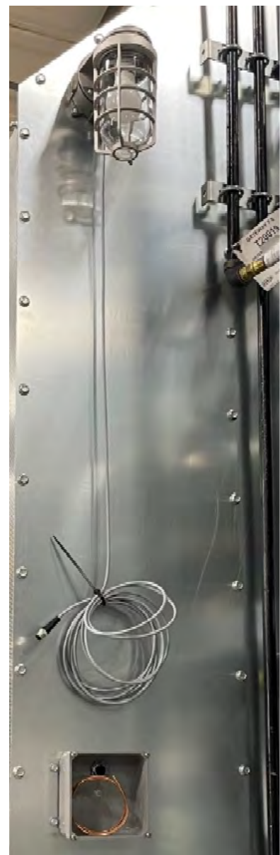
Image 11 - Work light cable & column over-temp capillary on front of cross-flow dryer
