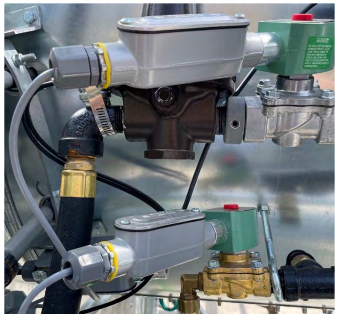
Image 6 - Cable connections to solenoid junction boxes
