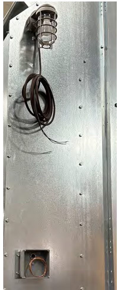
Image 11 - Work light cable & column over-temp capillary on front of cross-flow dryer
