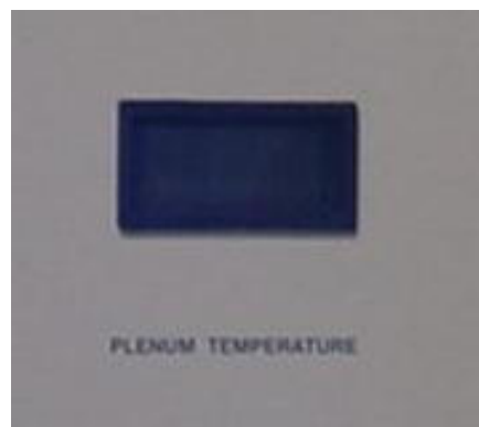
Figure 2.6a: Plenum Temp Display
