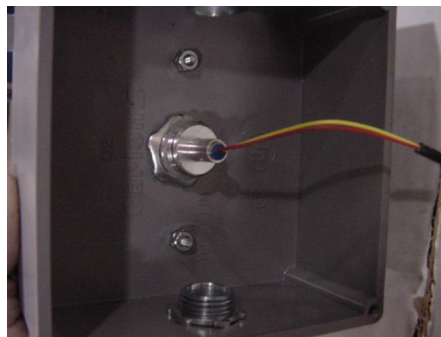
Photo 1.13: RTD sensor installation
