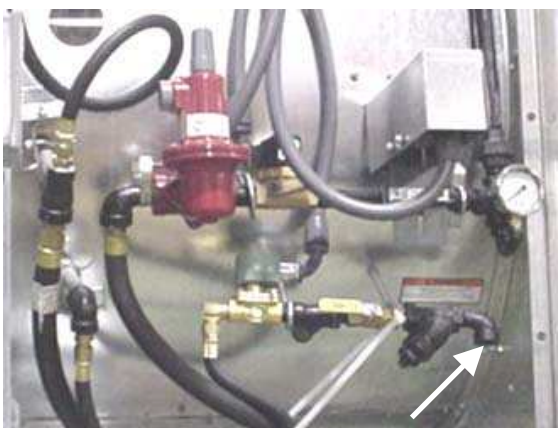
Connection to liquid manifold on Dryer
