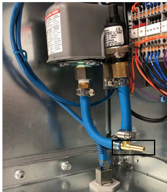
Image 4 – Air hose nozzle in power box
